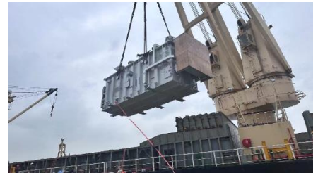
Philippines Visayas Substation Upgrading Project
