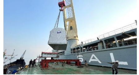
Bangladesh Rupsha 800MW CCPP Project
